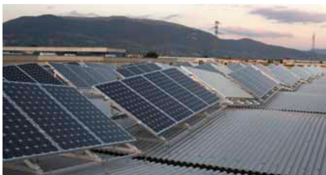
Bastia Umbra (PG) 46,08 kWp
