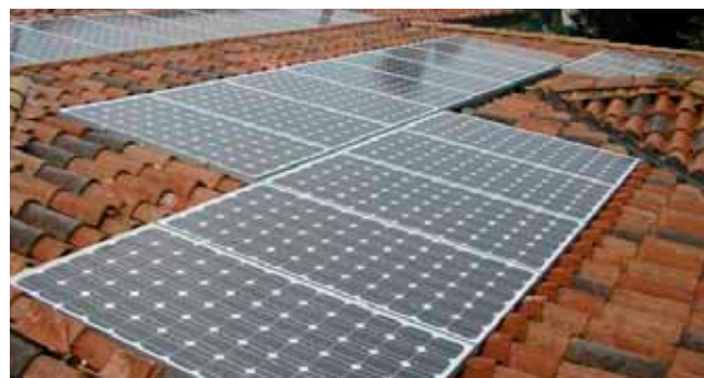
Rivoli (TO) 2,96 kWp
